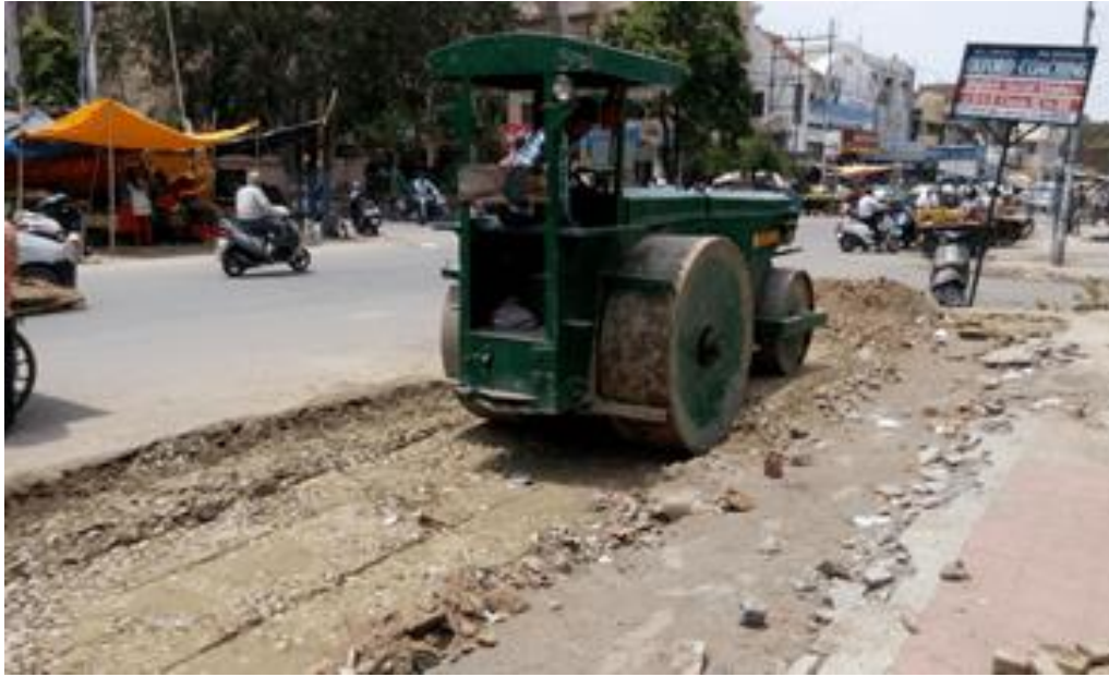
Figure 13. An ordinary road roller is being used to compact the WMM surface.
