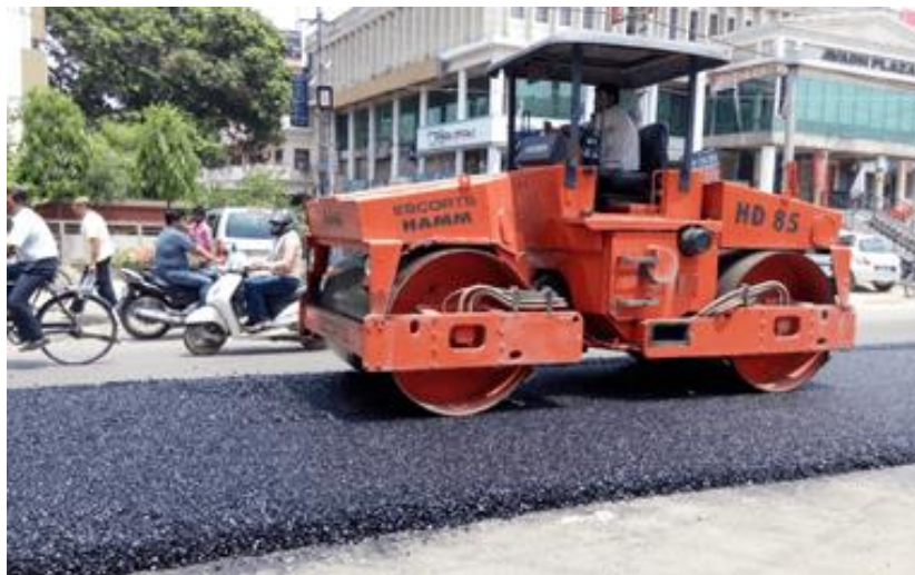
Figure 14. A vibratory roller is being used to compact the bitumen macadam surface.
