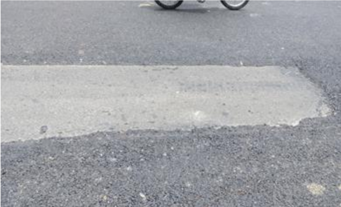
Figure 5. Gap left for the divider to be made after spreading the Bitumen Macadam
